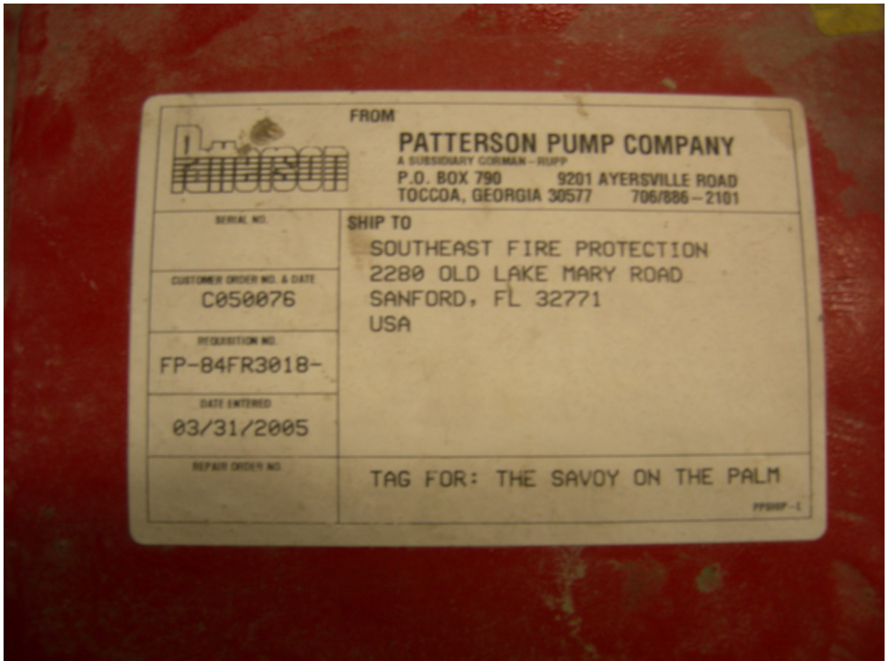
Figure 2.1.7 Fire Pump Installation label
