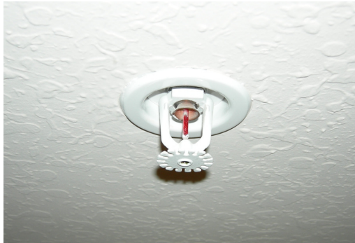
Figure 2.1.2 Savoy Unit Ceiling Sprinkler Head-Typical
