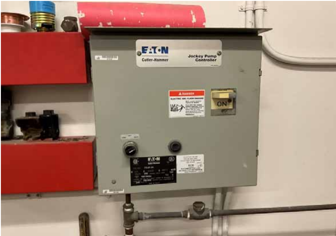
Fire Jockey Pump Controller
