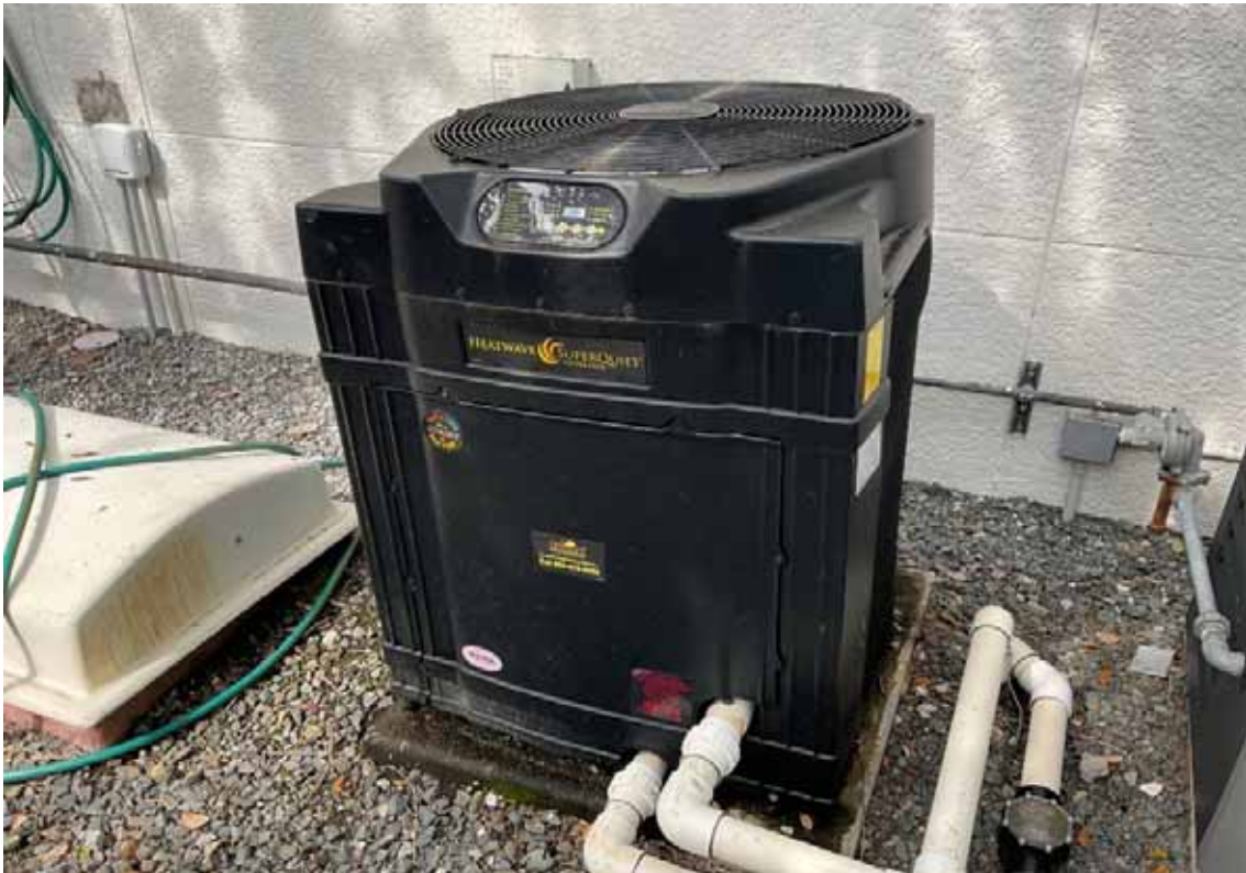
Spa Equipment, Heater
