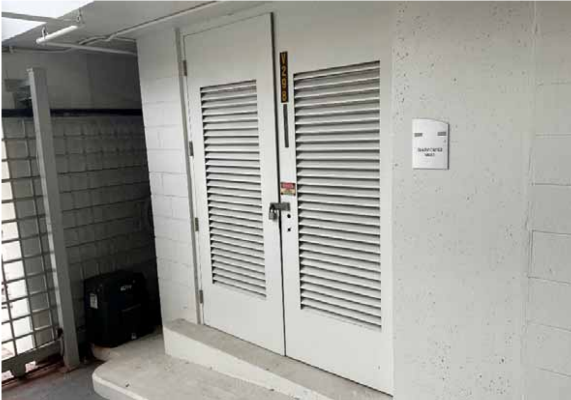
Doors - FPL Vault
