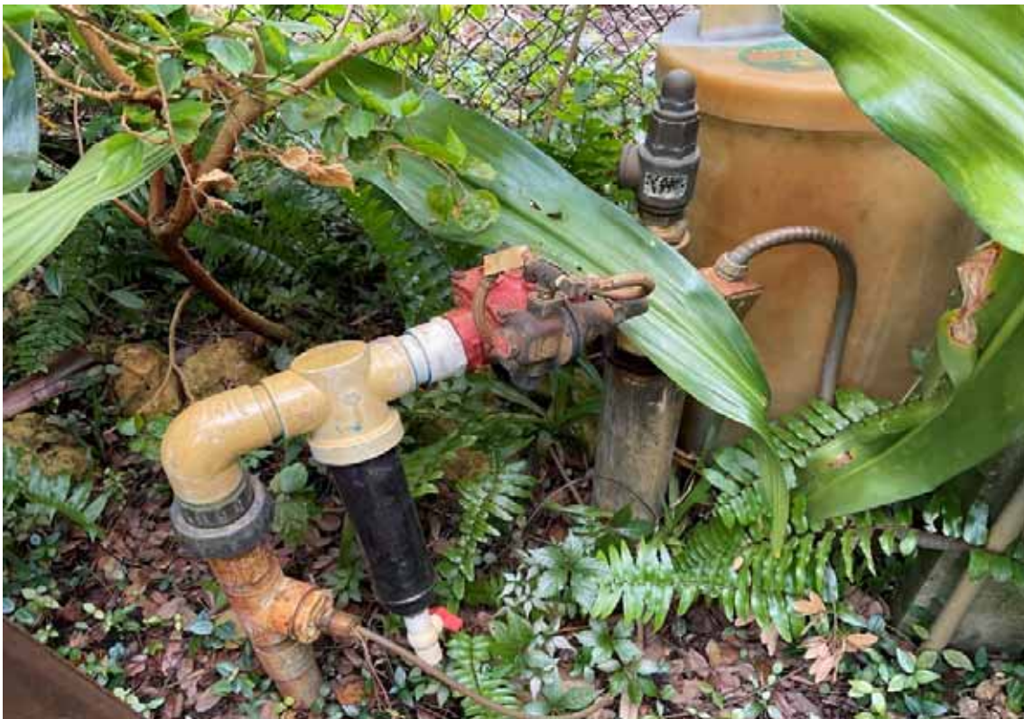
Irrigation Well Pump Station
