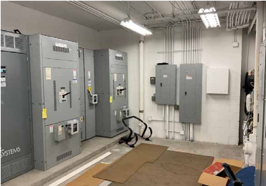
Main Electrical Room
