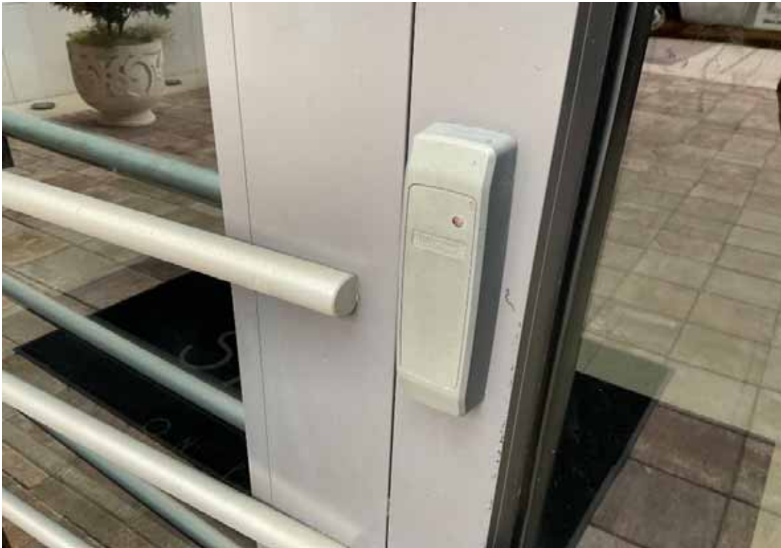
Access Control - FOB Reader
