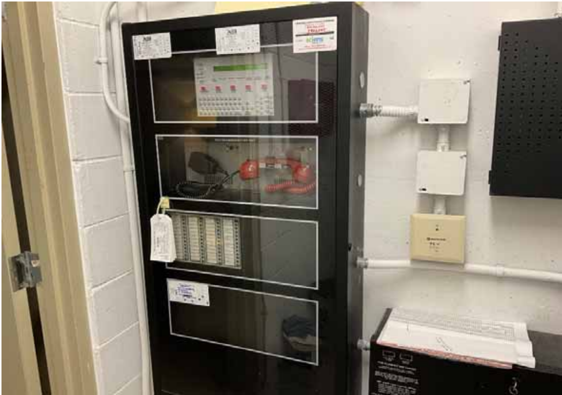
Fire Alarm Panel
