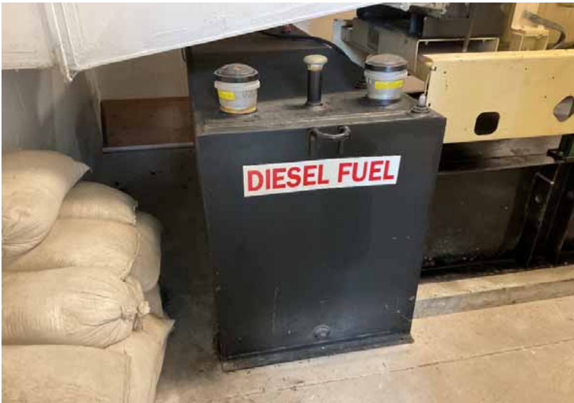
Generator Fuel Tank
