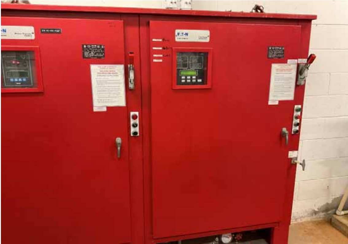
Fire Pump Controller
