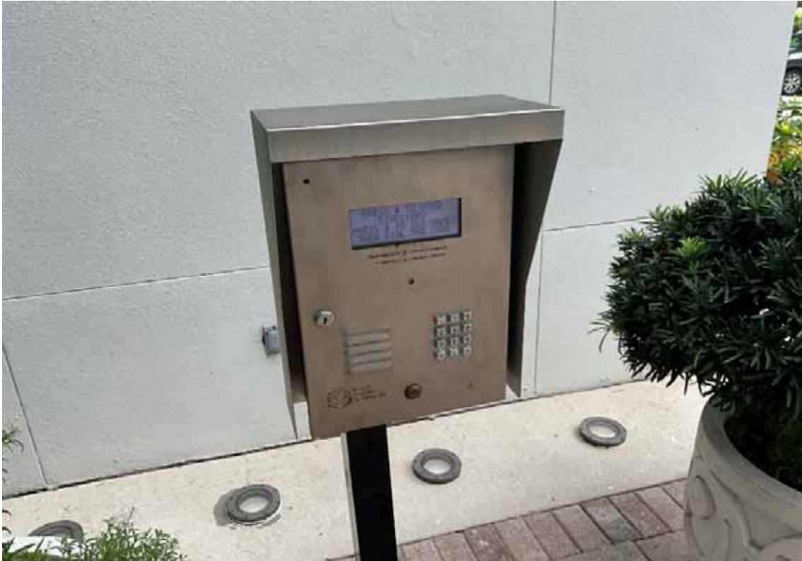
Access Control - Enterphone Panel
