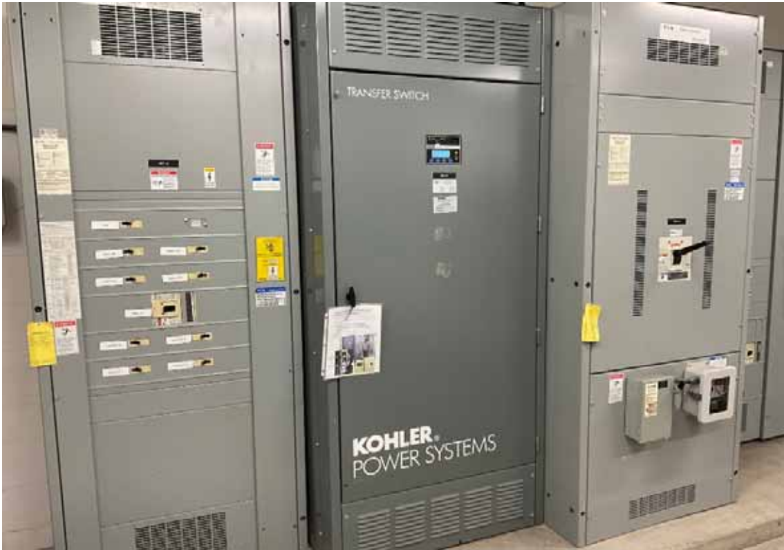
Generator Transfer Switch
