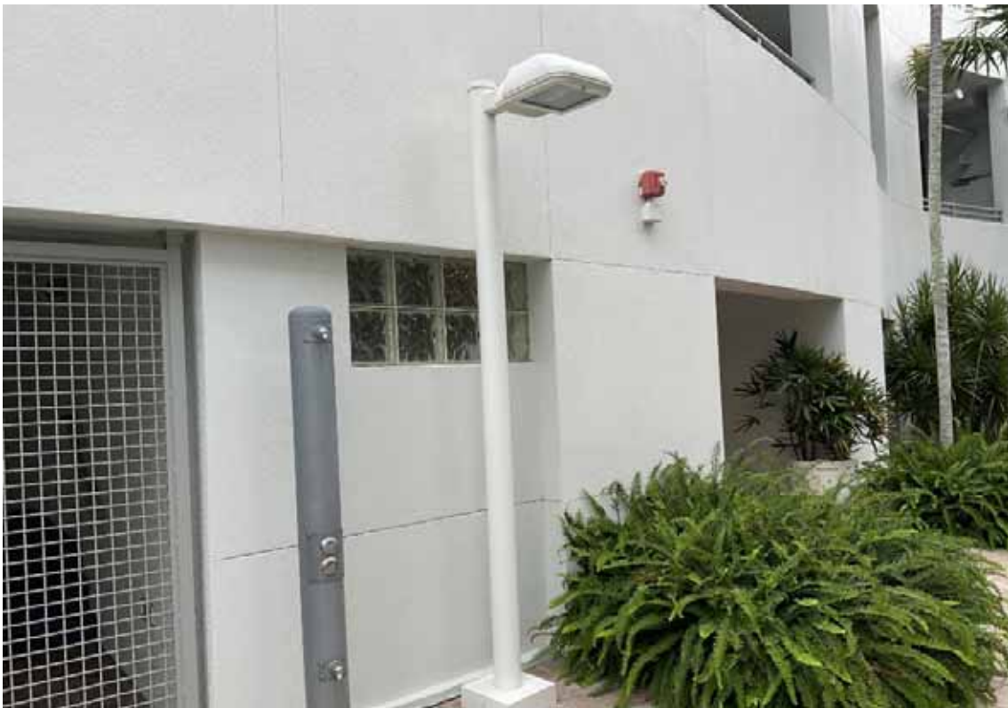
Light Pole & Fixture - Pool Deck
