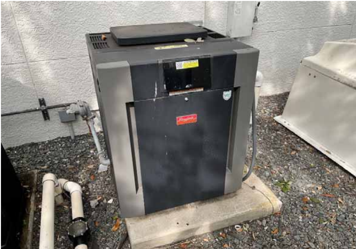
Pool Equipment, Heater
