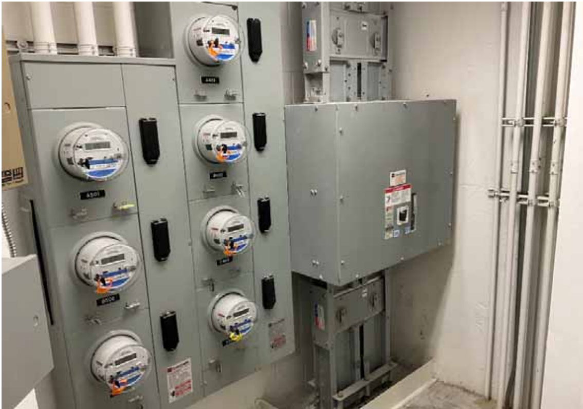
Electrical Meters & Panels
