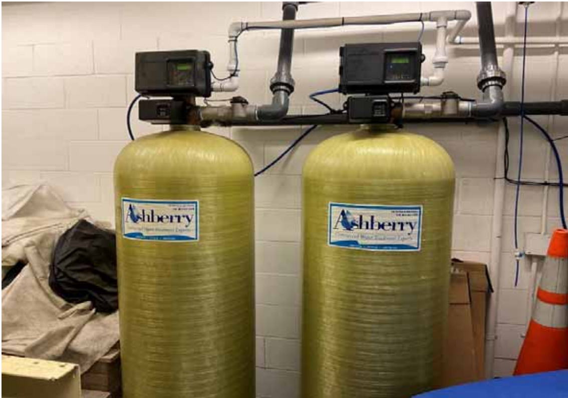
Water Softening System
