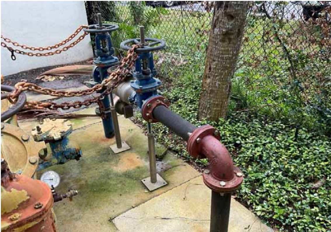
Backflow Preventer - Domestic Water
