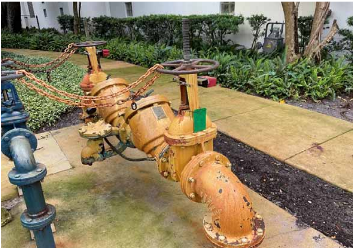
Backflow Preventer - Fire
