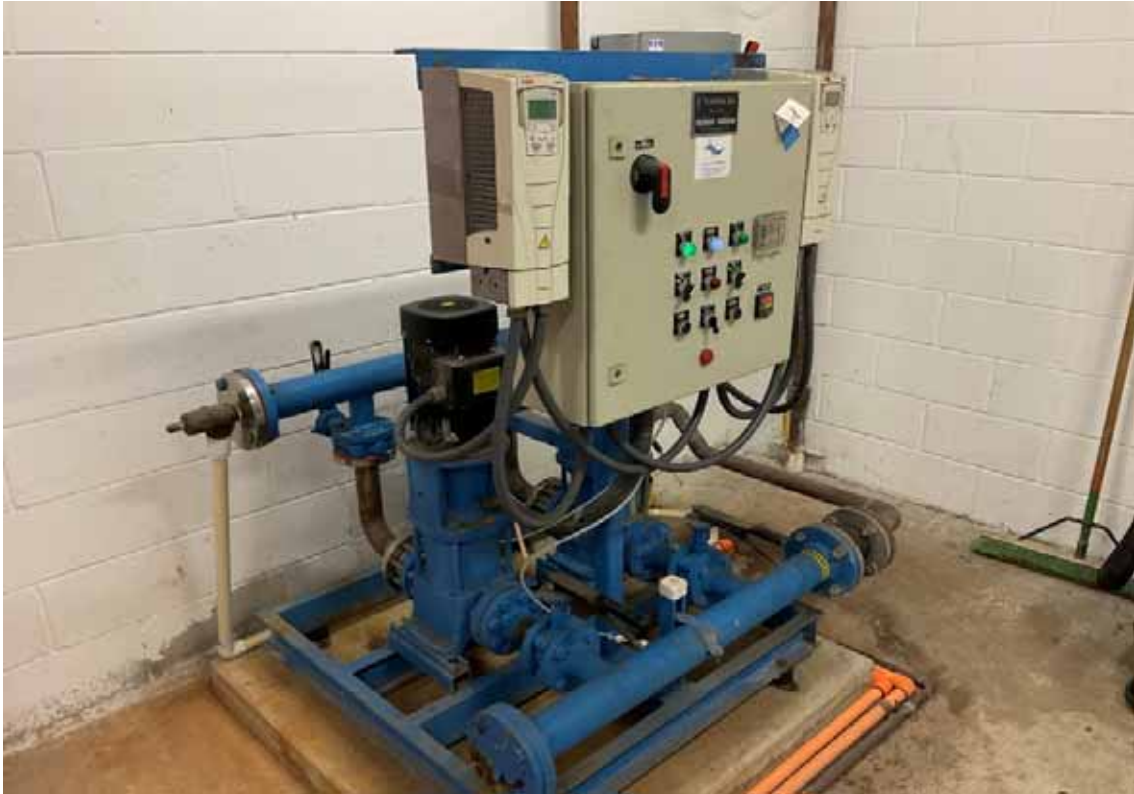
Domestic Water Booster Pump System
